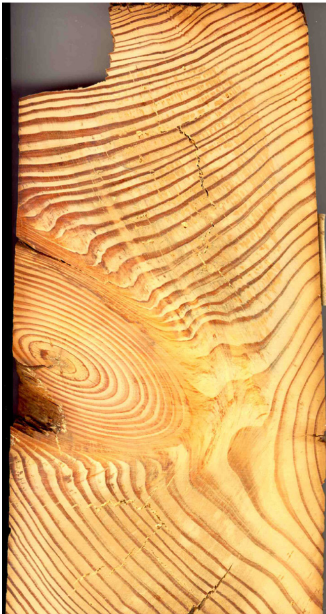
Fig. 1: This conifer ceiling beam ( Pinus sylvestris ) was inspected visually and with the help of an endoscope. No decay was found. Some weeks later the beam broke and two carpenters fell down one level, luckily not heavily injured. Later, a detailed analysis of the beam showed that there was a brown rot in an early stage in the center the cross-section. Obviously, strength was significantly lowered. On the sawn cross-section it was impossible to identify the decayed area. Surface sanding and microscopic analysis was required.
